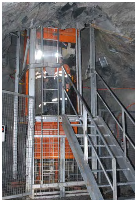
ALIMAK LIFT IN REWARD SHAFT
