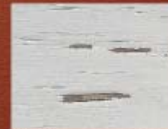
Moisture causes wood to shrink and swell, which causes paint to crack and flake off.
