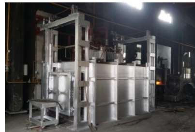
Conversion to Natural Gas + Fuel System Upgrade
