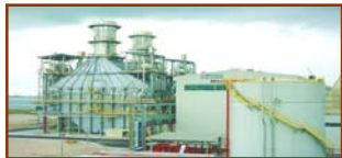
500MW Cogen Plant Operational: 2Q'07
