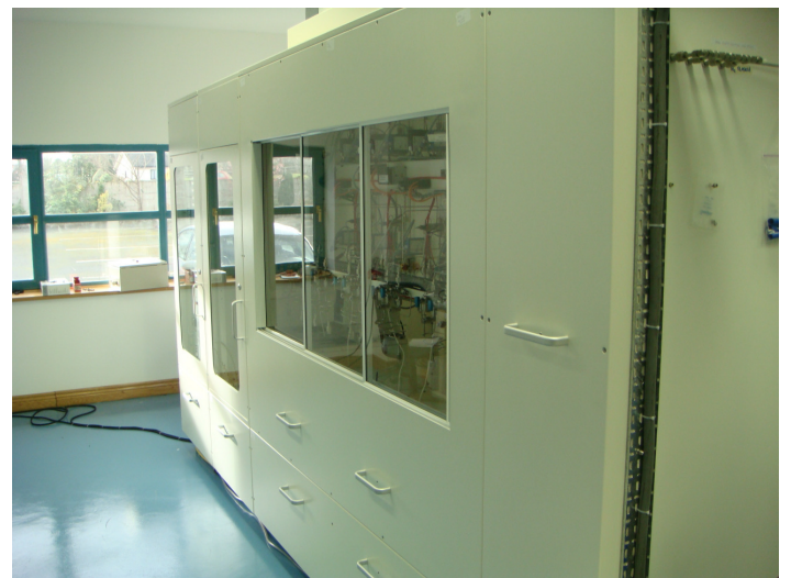
Gas Supply Unit
