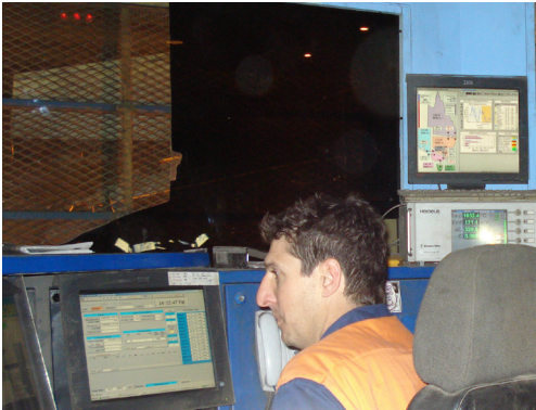
This photo depicts the main control room for the furnace operations at the Sydney Steel Mill. In the centre of the picture is a computer screen that monitors electricity prices for the eastern seaboard. At times of high electricity prices, OneSteel has the ability to interrupt production and sell the energy into the New South Wales power grid.
