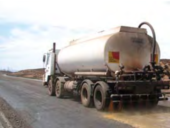
Water carts carrying recycled water combined with Dustreat (a natural dust-binding agent) are used to suppress dust on roads around Whyalla.
