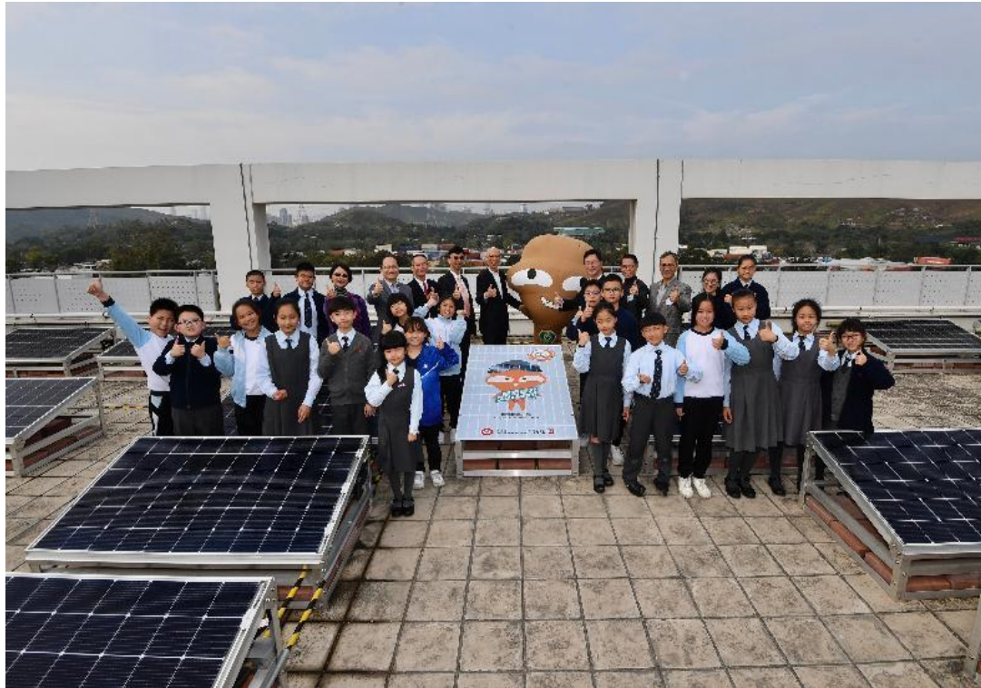
Photovoltaic systems in more than 100 schools and NGOs Contract sum: HK$ 19M
