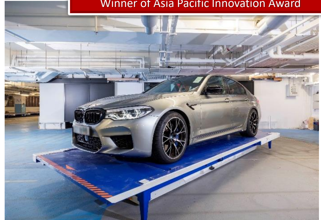
Hong Kong's First Automated Robotic Parking System Contract sum: HK$ 12M
