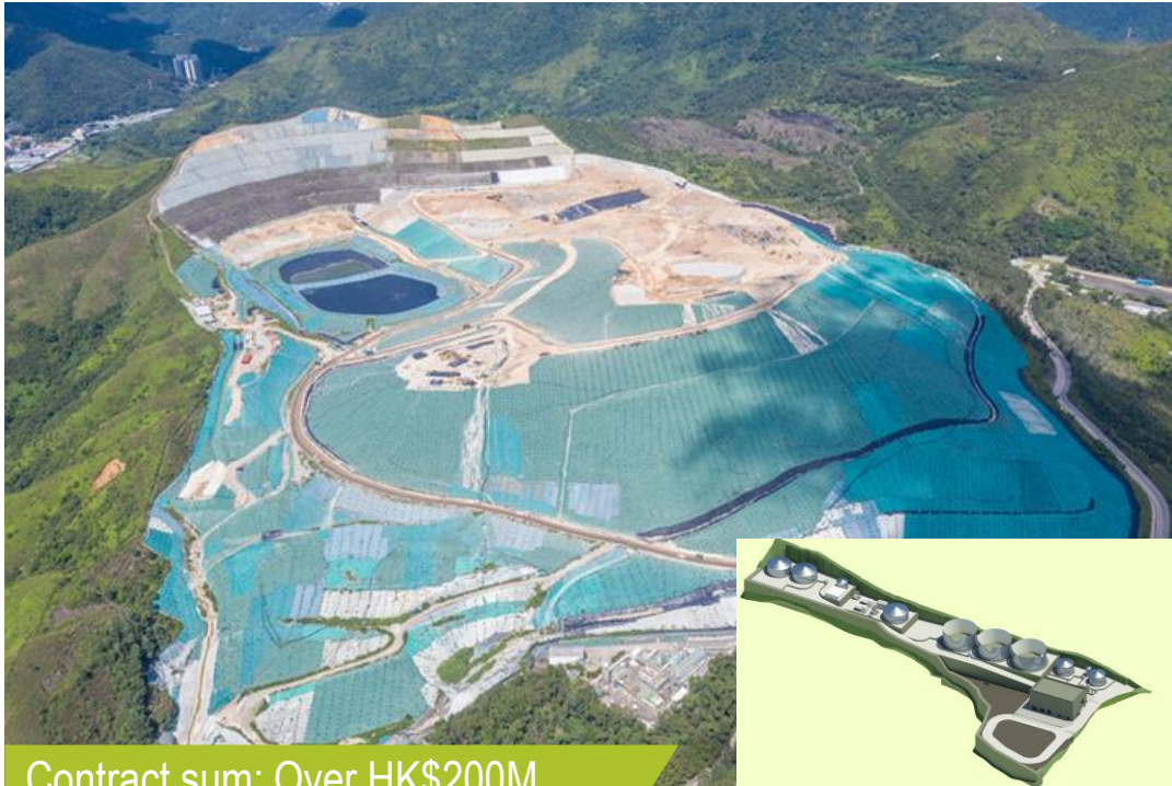
New Leachate Treatment Plant for North East New Territories Landfill Extension (NENTX)
