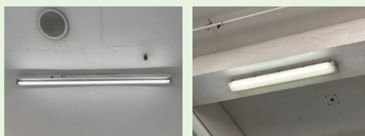
LED lighting in the corridor and the parking lot of Tsing Yi Property
