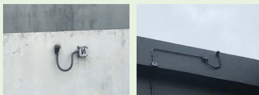
Light sensors at the rooftop and 9/F of Tsing Yi Property
