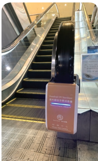
UV light escalator handrail cleaners installed to inhibit germs and viruses on escalator handrails 在扶手電梯安裝紫外線消毒殺菌器以抑制細菌和病毒滋生
