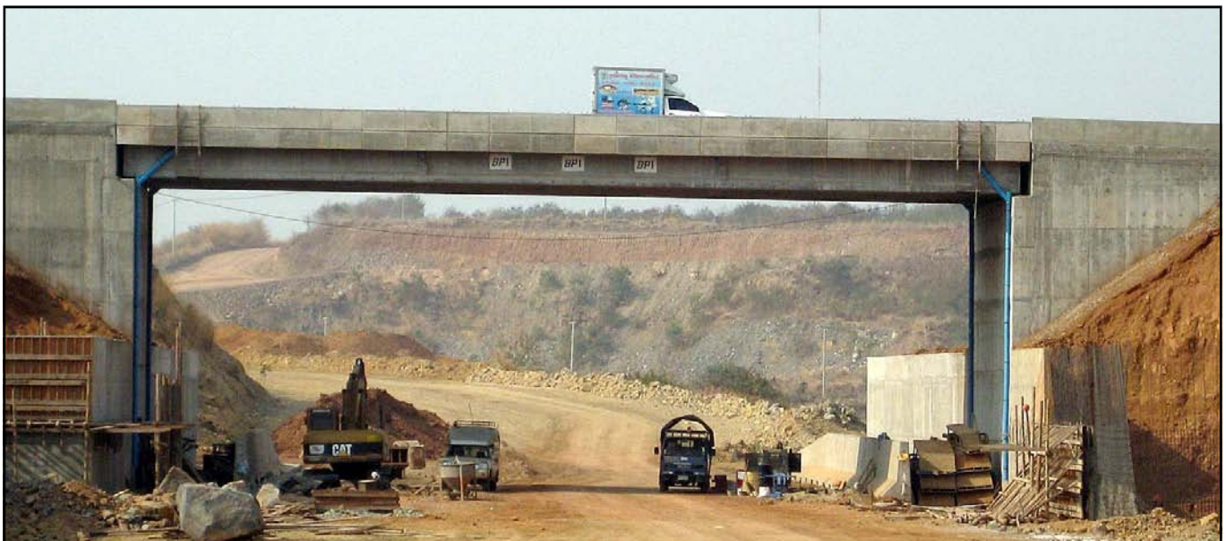
View of the Underpass from Chatree North, final work on the "wings" almost completed.
