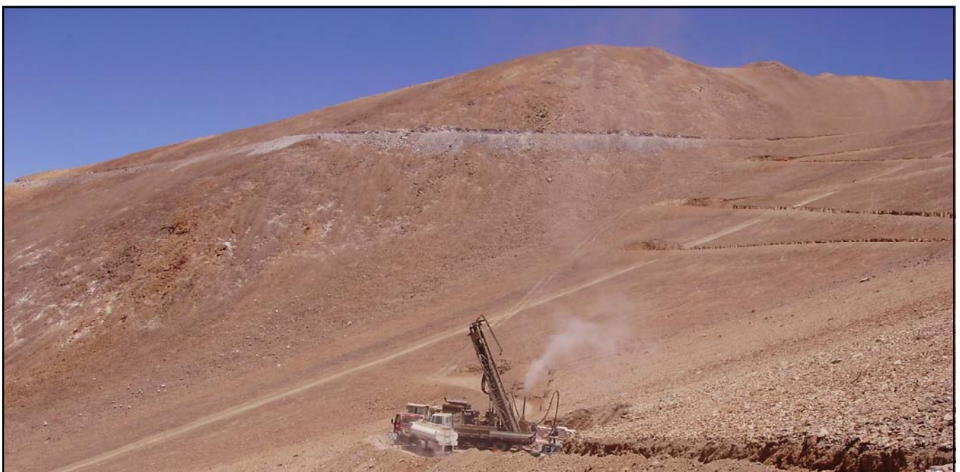
Drilling on Arqueros Prospect, Nueva Esperanza Project, Chile showing terraced drillpad complex.
