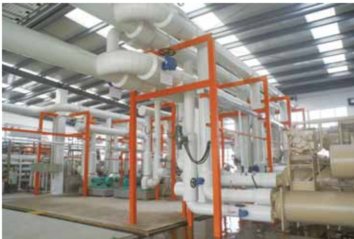
Zibo Waste Water Source Heat Pump Project 淄博污水源熱泵項目
