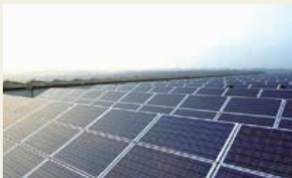
Suqian Rooftop Solar Photovoltaic Energy Project 宿遷屋頂太陽能光伏發電項目
