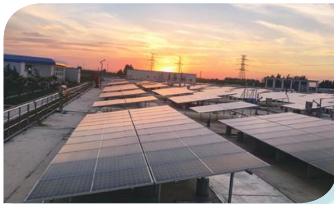
In-plant solar photovoltaic facilities in Zibo Waste Water Treatment Project (Plant 1) 濰博污水處理項目（一廠）的廠內光伏設施
