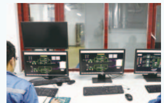
Control room setup
