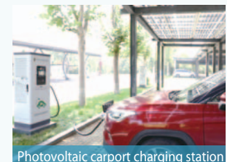
Photovoltaic carport charging station
