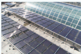
Solar water heating system
