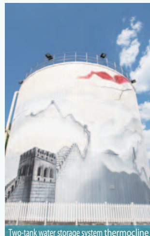
Two-tank water storage system thermocline
