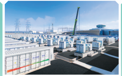
Large-scale energy storage project
