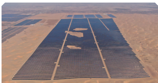
Photovoltaic Sand Control Project
