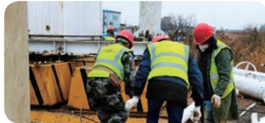
▲ Securing power generation of Wuhan Huoshenshan Hospital
