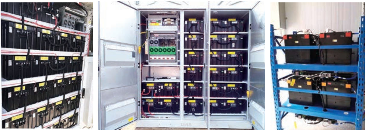
▲ Recyclable use of power battery site at the base stations
