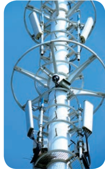
▲ Infrared night vision cameras installed on towers
