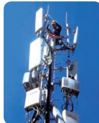
▲ IoT collection equipment placed on towers
