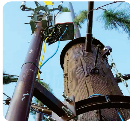
▲ IoT antenna at Yellow Crane Tower
