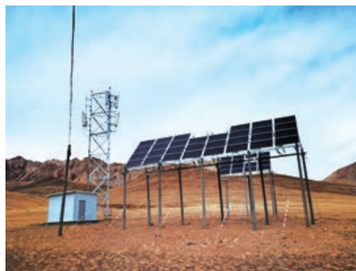
▲ A photovoltaic communication base station in Rikaze
