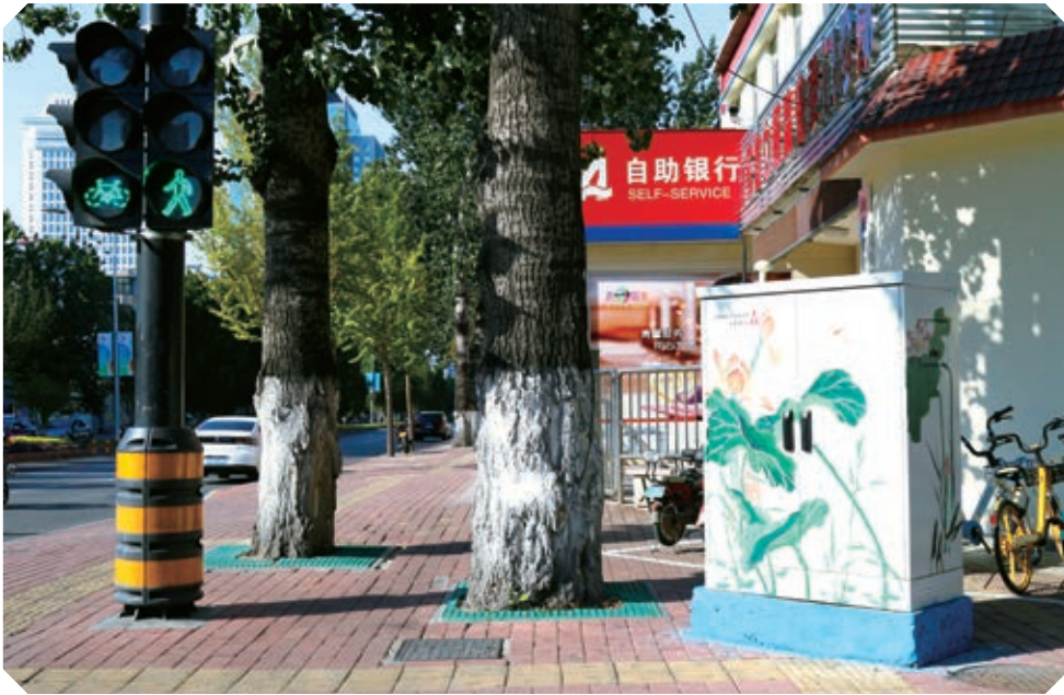
▲ Traffic signal light power backup cabinet
