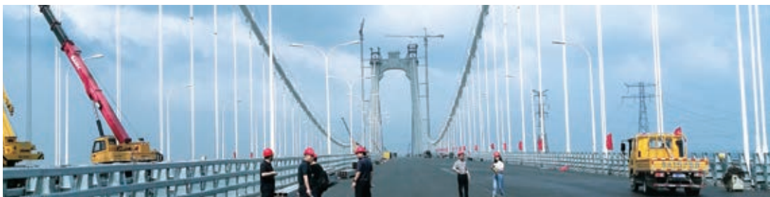
▲ Shared use of street light poles and single-tube towers
