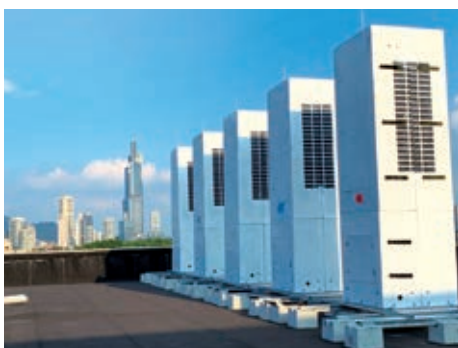
▲ Deployment of 5G facilities on the rooftop of Jiangsu Provincial CCP Committee
