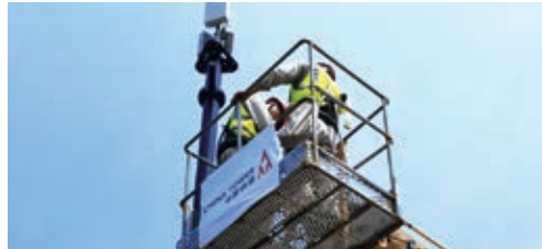
▲ Improving 5G coverage in core areas by using city integrating local poles
