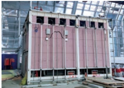
▲ Deploying antennas in built-in structures in the station
