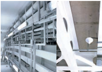
▲ Distributed antenna inside the building
