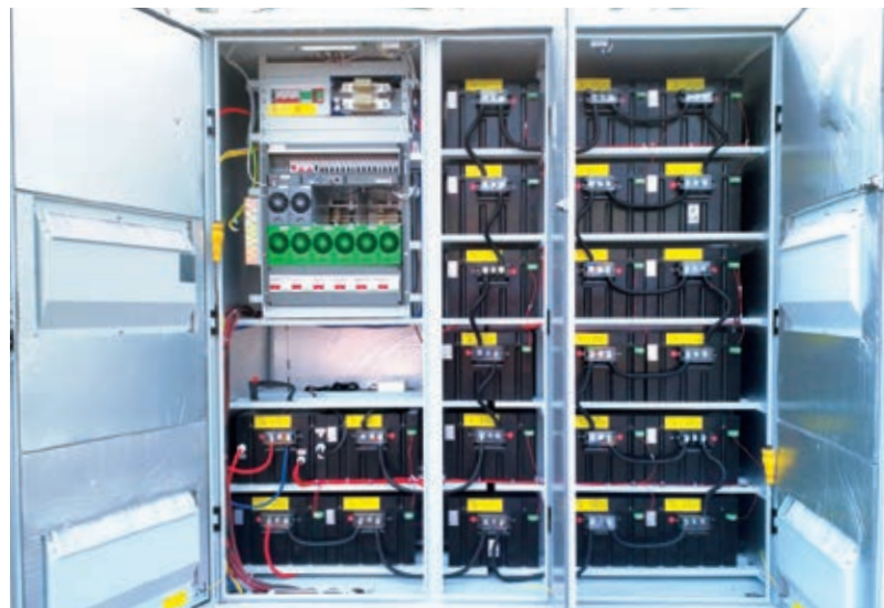
▲ Application of lithium titanate battery
