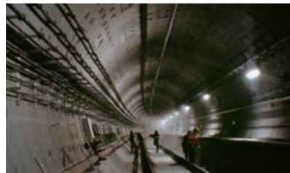
▲ Layout site of leaky cables in subway
