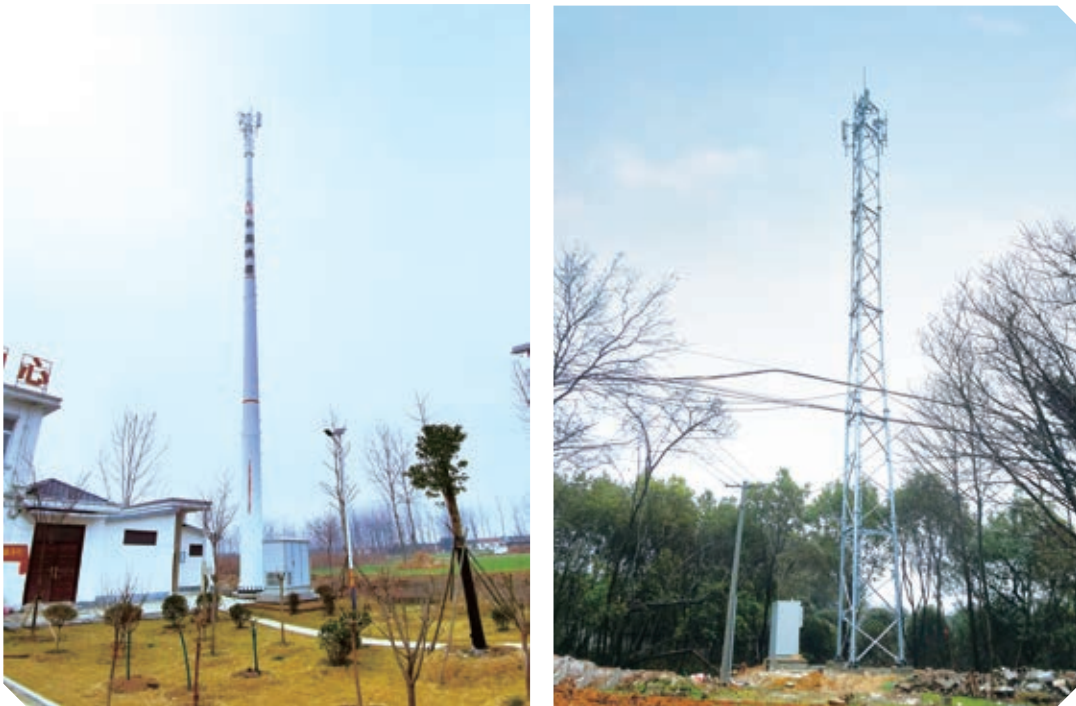
▲ Application examples of structural mast innovations
