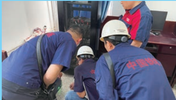
Power security operation
