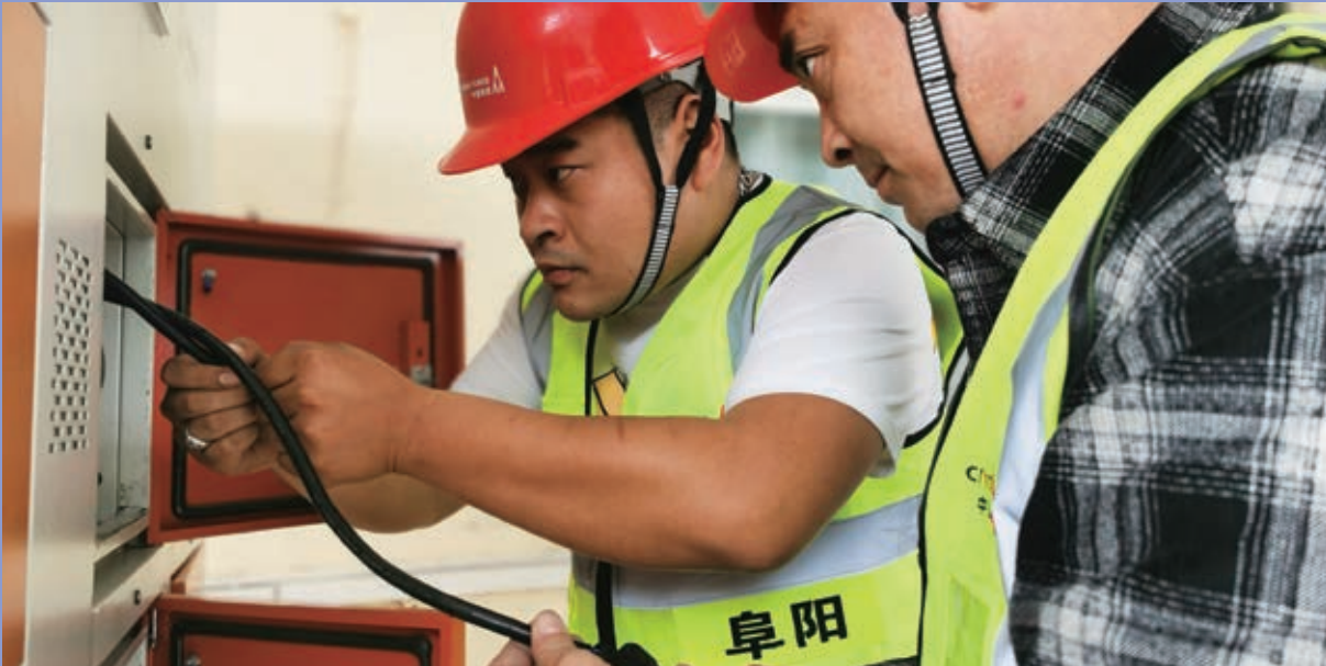
Identification of potential risks for battery exchange cabinets
