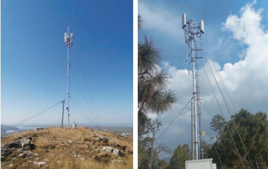
Example of low-cost guyed mast application
