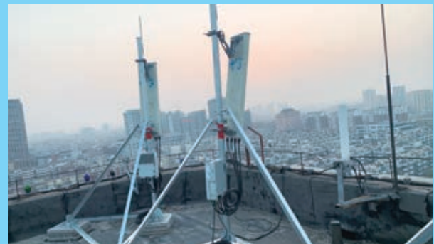
Deployment of 5G facilities on the rooftop of the office of Jilin Provincial Department of Industry and Information Technology
