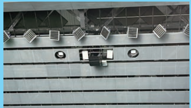
Internal Infrastructure in the Capital Gymnasium
