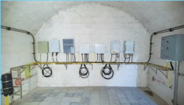
Sharing railway tunnel cabinets
