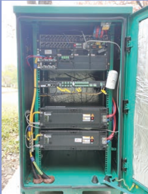
Site for application of modular power supply
