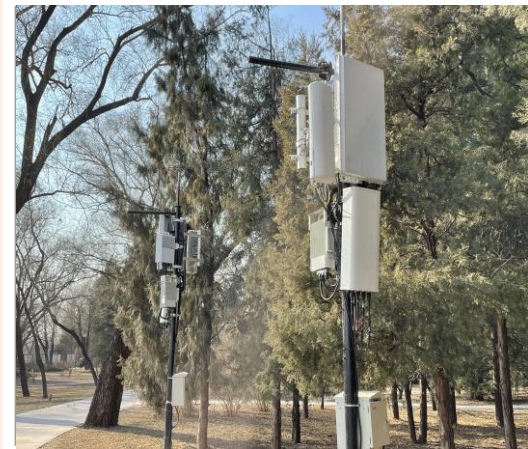
Constructed 5G network by sharing of social resources
