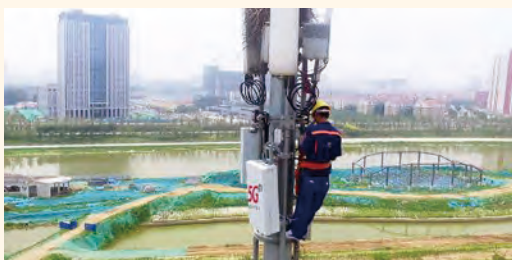
5G base station maintenance
