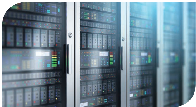
Data centres equipped with energy saving technology
