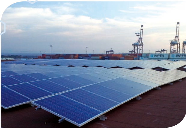
Solar array at Hutchison Ports Mexico
