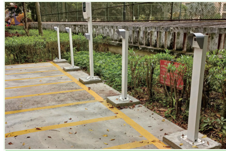
Electric vehicle charging piles
