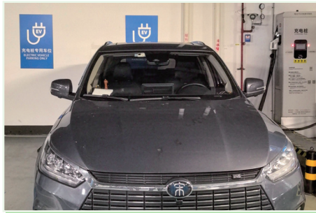
Electric vehicle charging piles
