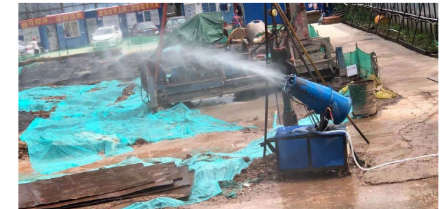
Sprinklers and covers
