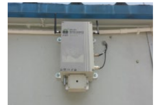
Noise and dust monitoring system
