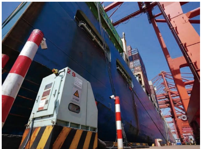
The power supply system of the comprehensive energy-saving gantry cranes in Tianjin Container Terminal.
