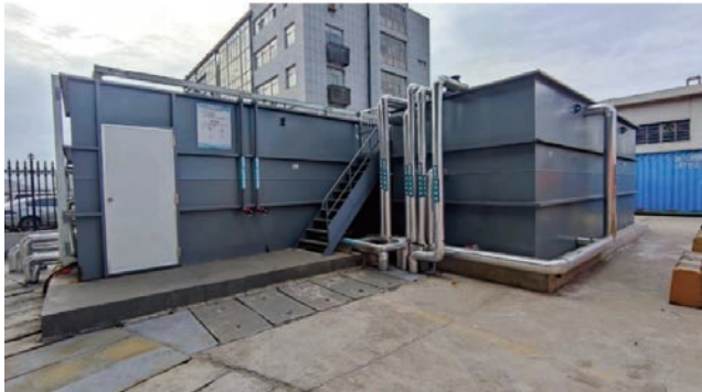
The sewage treatment station in Lianyungang New Oriental Terminal is used to treat and purify the sewage to achieve the discharging standard or reuse.
