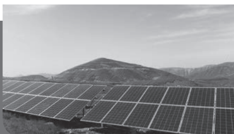
Centralised Photovoltaic Power Plant, Qixian Miaokou, Henan Province
