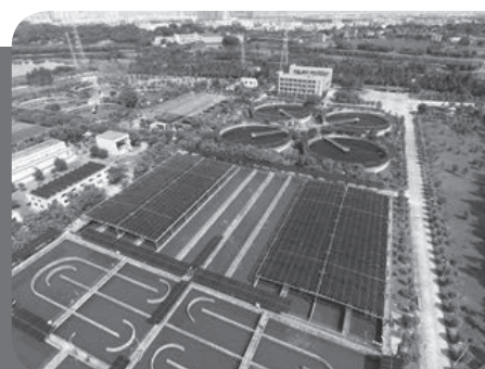
Distributed Photovoltaic Power Station in a water plant of BEWG, Dongguan, Guangdong Province
