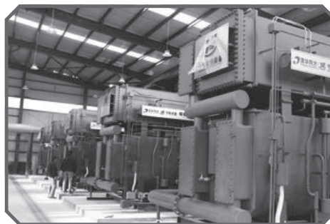
Clean coal consumption and power plant excess heat energy centralised heat supply project in Yinchuan City, Ningxia Hui Autonomous Region
