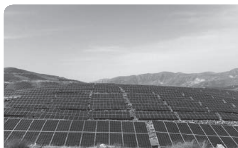
Centralised Photovoltaic Power Plant, Qixian Miaokou, Henan Province
