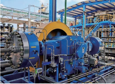
Hydrogen compressor for loading in mother station
