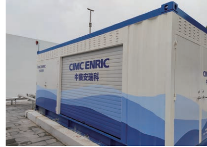
Hydrogen compressor in hydrogen refuelling station
