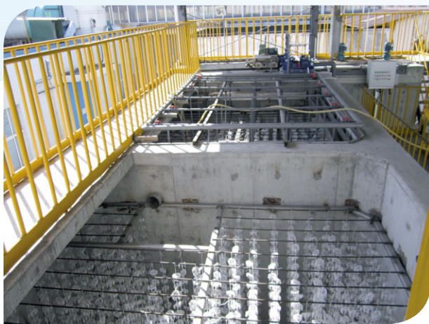
Spray paint effluent treatment facility
