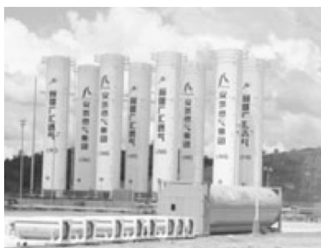
Cryogenic liquid vacuum storage tank Manufacturer: the Zhangjiagang Group
