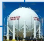
液氢储配站 Liquid H2 distribution station
