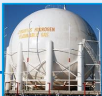
液氢储罐 Liquid H2 tank
