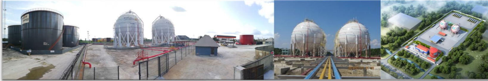
Above: Delivery of multiple large spherical tank projects in Thailand, Ghana, Nigeria and other places
