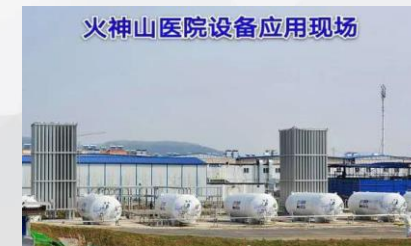
Above: We supported the fight with epidemic by providing liquid oxygen storage tanks with Anjieshui intelligent device installed
