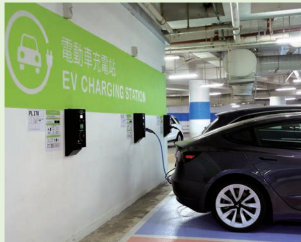
EV chargers are provided at +WOO car park
