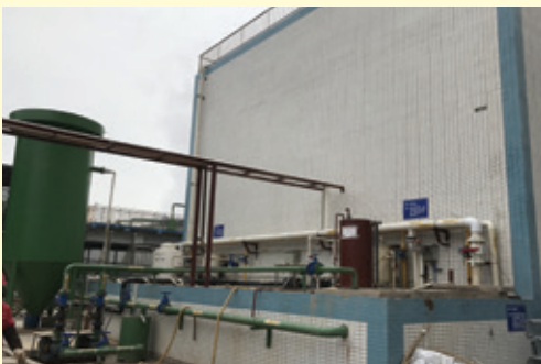
重慶康樂製藥有限公司處理廢棄物設施 — 厭氧池 Waste disposal facility of Chongqing Kangle Pharmaceutical Ltd. — Anaerobic digestion tank
