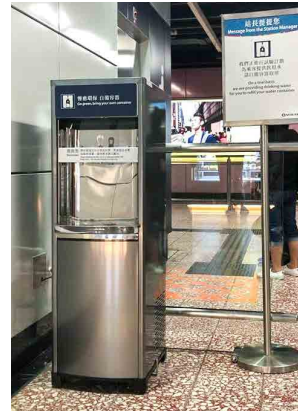
Drinking water dispenser at Prince Edward Station
