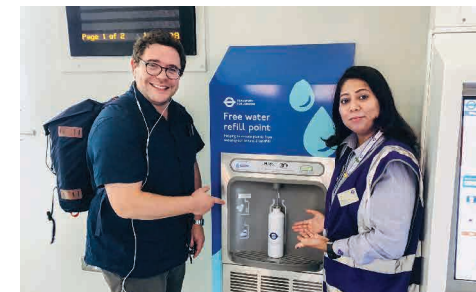
Eco-dispenser at Brentwood Station
