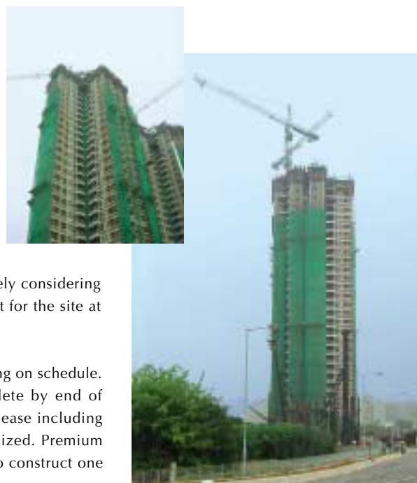
Fanling Sheung Shui Town Lot No. 189 55% owned by the Group, the construction work of this site is underway for three 40-storey residential towers. Total gross floor area of the development will achieve approximately 45,120 sq.m. with 139 carparking spaces.
