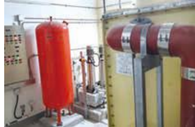
Rainwater Collection System
