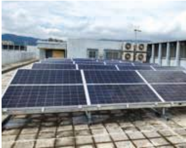
Solar Panel at Rooftop
