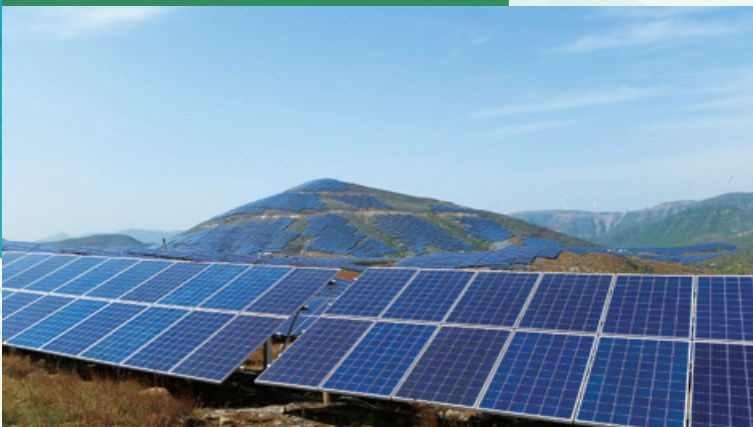
Centralised photovoltaic power plant, Qixian Miaokou, Henan Province 河南省淇縣廟口集中式光伏發電站
