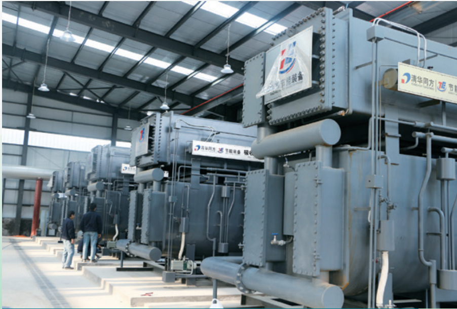
Clean coal consumption and power plant excess heat energy centralised heat supply project in Yinchuan City, the Ningxia Hui Autonomous Region 寧夏回族自治區銀川市清潔化燃煤及發電站餘熱能源集中供暖項目
