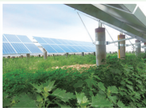
First agro-photovoltaic power project in Shanghe County, Shandong Province 山東省商河縣首個農業光伏發電項目
