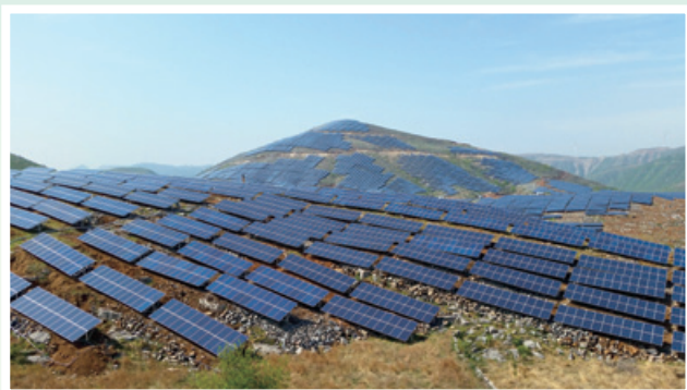
Qi County Miaokou Baisi Village Hillside Photovoltaic Power Plant Project 淇縣廟口鎮白寺村荒山光伏發電站項目
