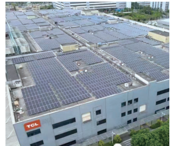
▲ Completion of TCL Communication's Photovoltaic Project
