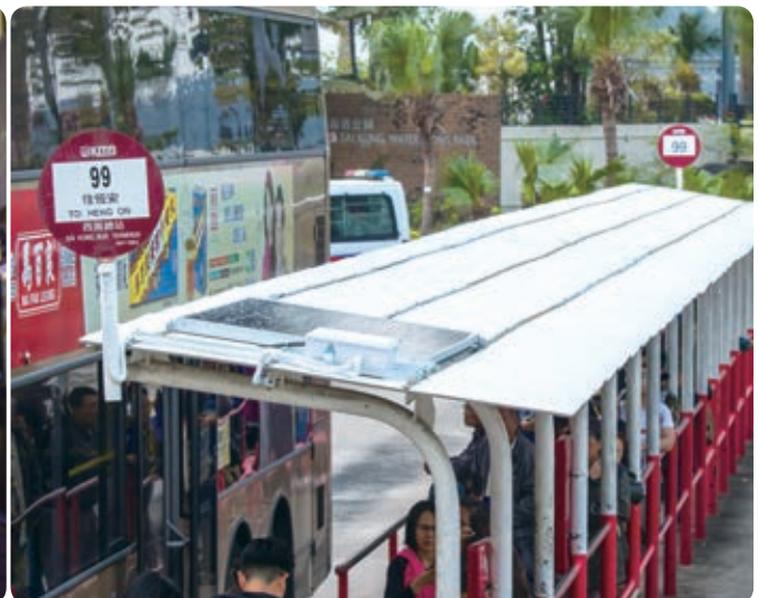
100 bus stops have been equipped with solar power equipment
