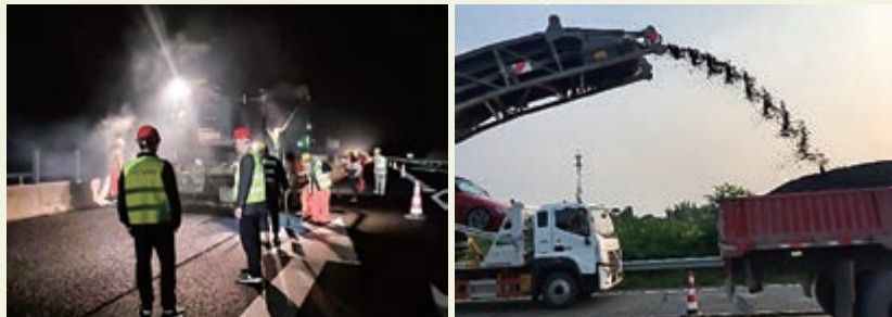
● NovaChip super-thin wear layer surface construction technology applied to reduce the pavement damage rate
