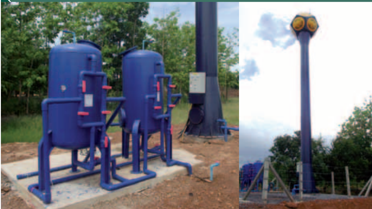
New water supply system for Klong Talad village, Phitsanulok Province.
