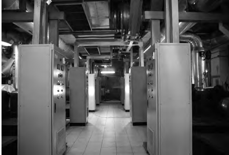
Figure 22: VSD panels for primary chilled water and condenser water pumps
