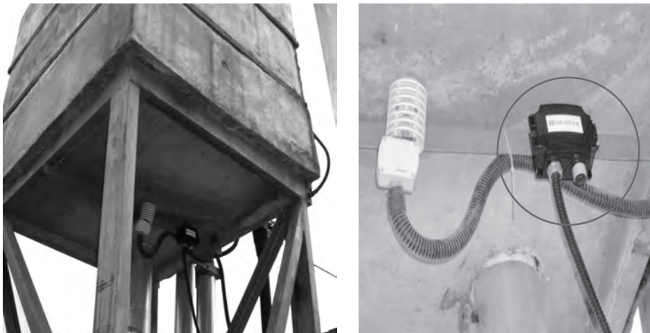
Figure 19: Outdoor temperature and humidity transducer (installed under the expansion tank on the building rooftop, in proximity to the cooling tower)
