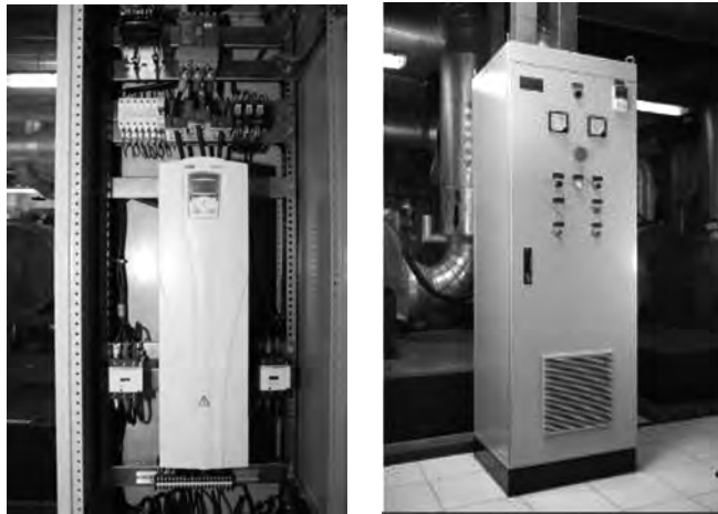
Figure 23: VSD panels for primary chilled water pumps
