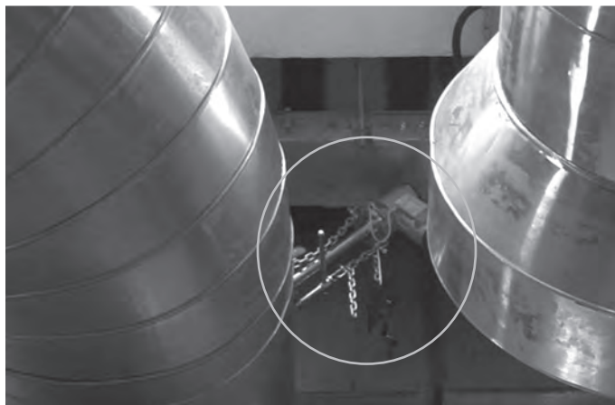
Figure 17: Electromagnetic flow meter installed on the secondary chilled water main return pipe
