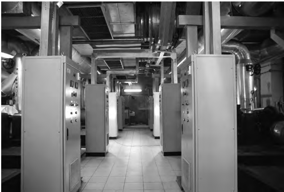
Figure 10: Chiller Plant at Corporate 1 Avenue
