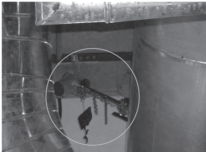
Figure 16: Electromagnetic flow meter installed on the primary chilled water main supply pipe
