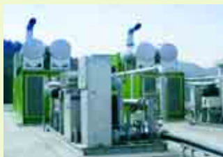
沼氣發電廠 Methane-to-energy plant
