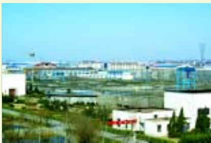
Zibo Northern Plant (Overall upgrade work in progress) 淄博北廠（全面升級改造工程進行中）
