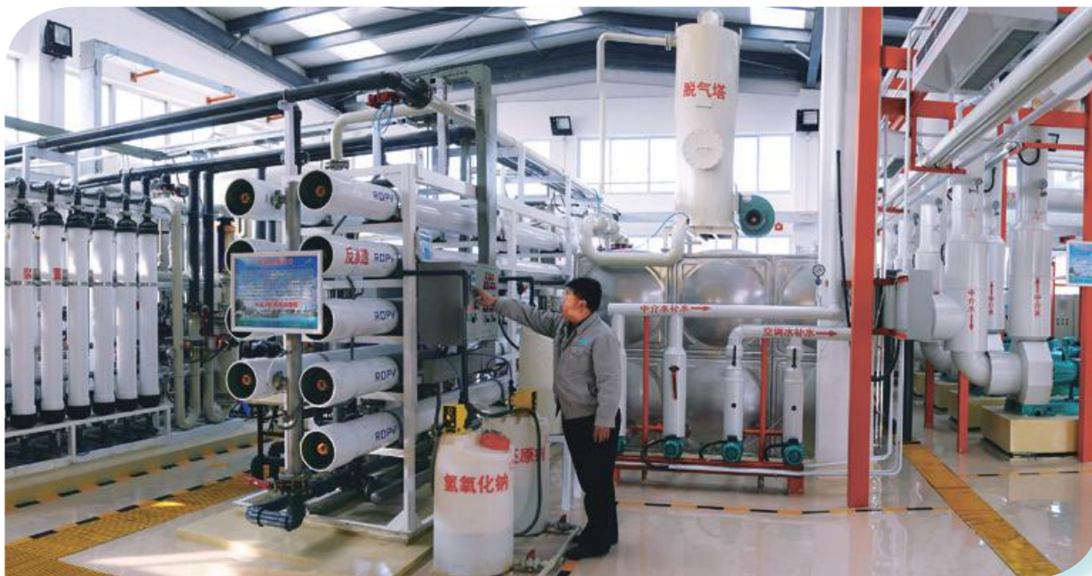
Zibo Waste Water Source Heat Pump Project 淄博污水源熱泵項目
