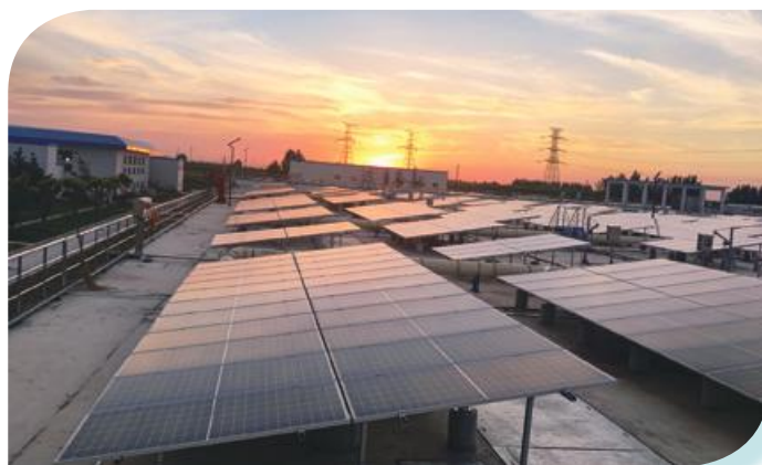
In-plant solar photovoltaic facilities in Zibo Waste Water Treatment Project (Plant 1) 濰博污水處理項目（一廠）的廠內光伏設施
