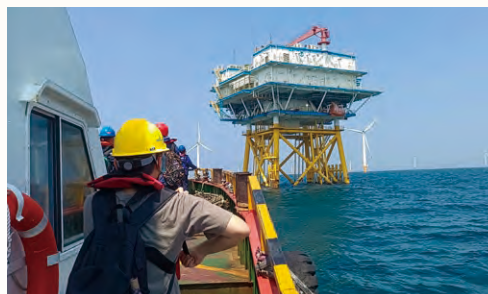
Construction of a 5G base station on the offshore wind power platform in Yangjiang City, Guangdong Province.
