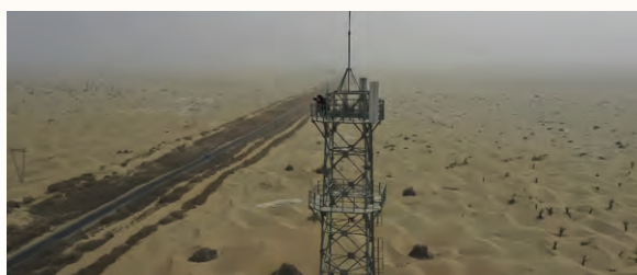
China Mobile launched the first 700MHz 5G ultra-long-range base station on a desert highway.
