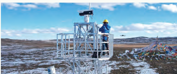
China Mobile’s base station at the source of the Yellow River.
