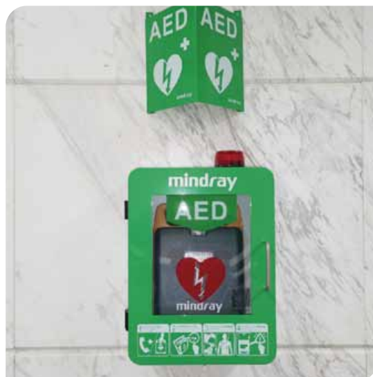
AED equipment was provided by Changshu Power Plant
